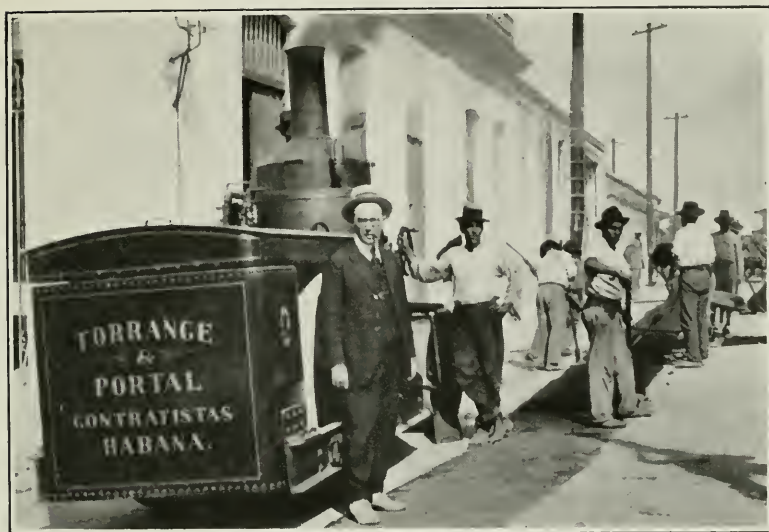
FIG. 12.—Paving Havana with something better than good intentions. The Barber Asphalt Paving Company furnishes asphalt and steam roller. In the foreground is Stanley H. Rose, Manager of Foreign Sales.
